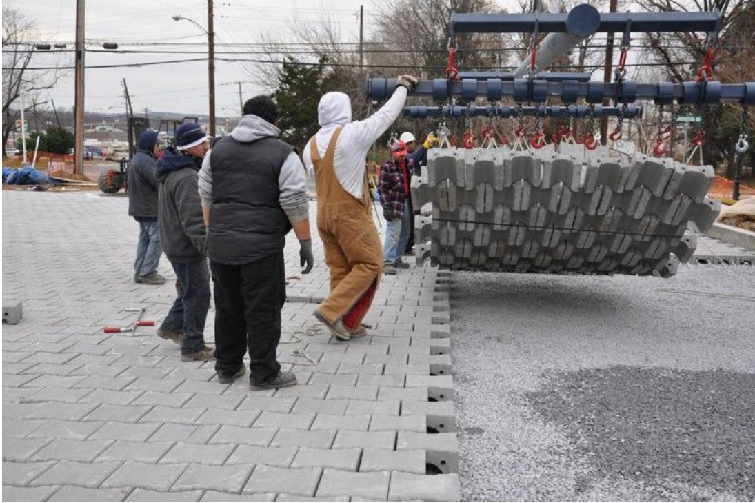
Installation at Bladensburg, Maryland Town-Hall parking lot during December 2010.
