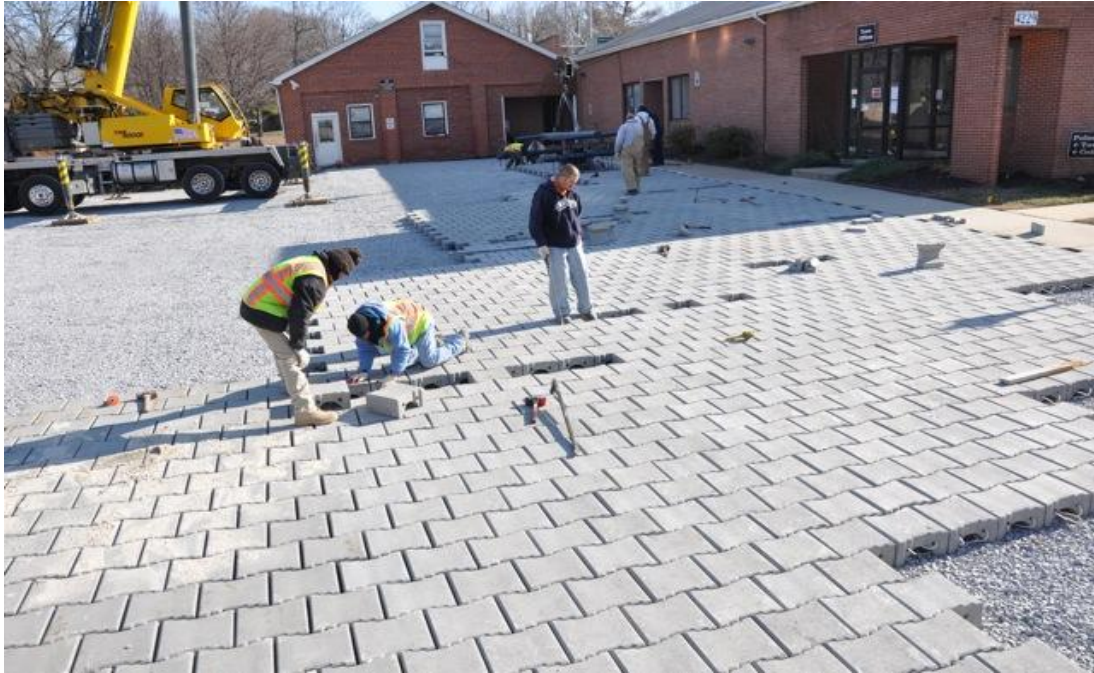
Installation at Bladensburg, Maryland Town-Hall parking lot during December 2010.
